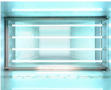
PUV-D UVC lamps in operation
